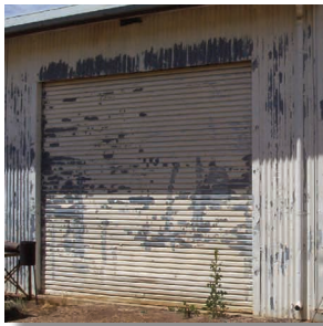
Lead in paint
